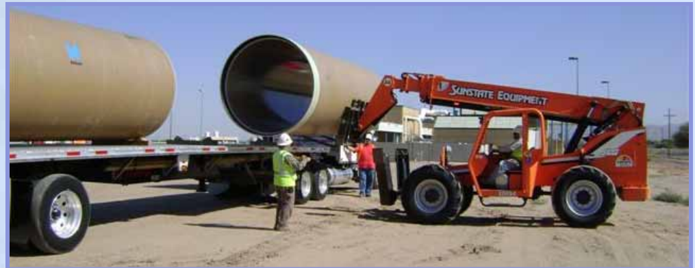
Plant Interconnect – Pima County, Arizona
